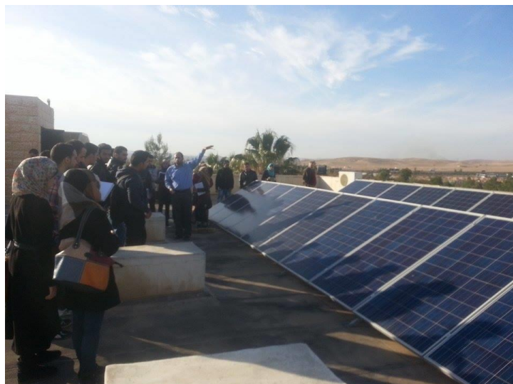
Figure 3: Fixed PV systems of 30 kW project at Presidency Building.
