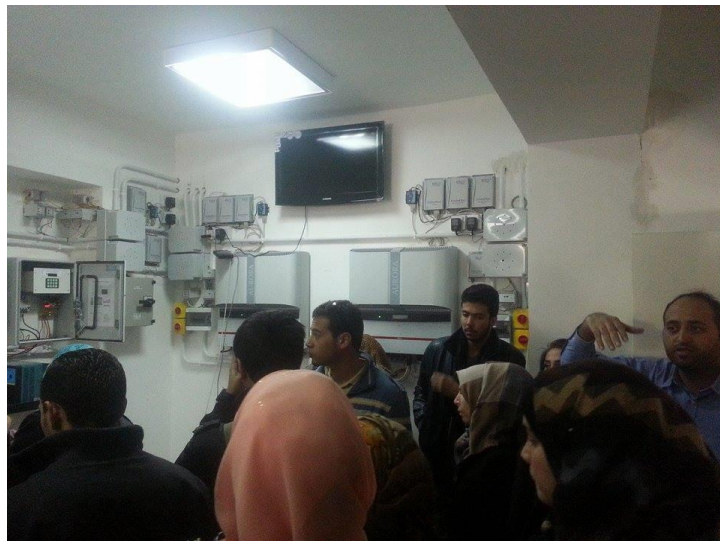
Figure 2: Control and monitoring room of 30 kW project at Presidency Building.
